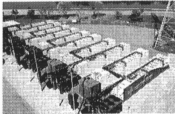
Grid-scale battery storage
